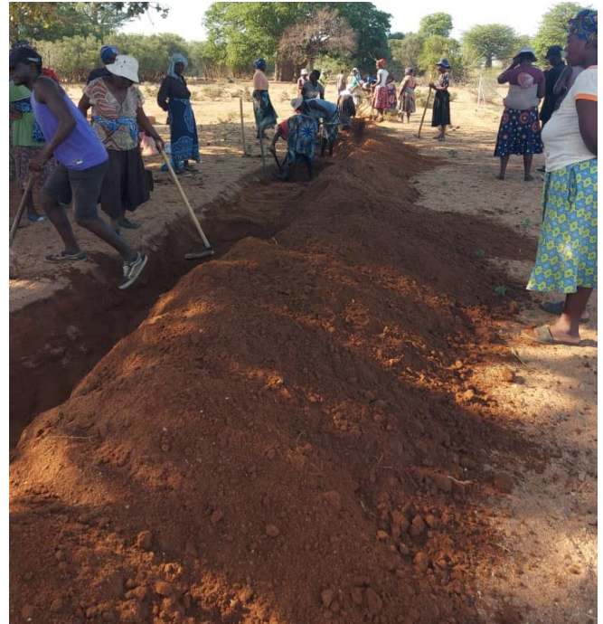
Above: Swale construction in Mutsiyo Village under Nyanyadzi River Watershed Management Project
