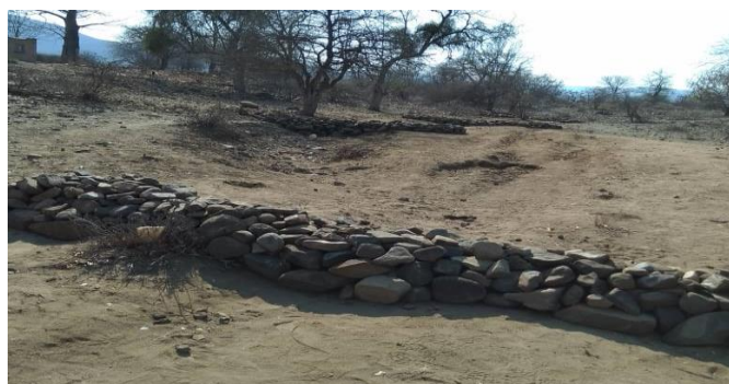
Pictures above: shows gabions being constructed by communities to along Nyanyadzi, Mvumvumu and Changazi rivers
